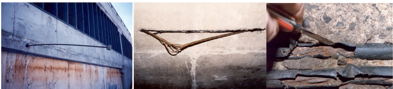
Figure 1: Examples of post-tension tendon failure due to corrosion.
